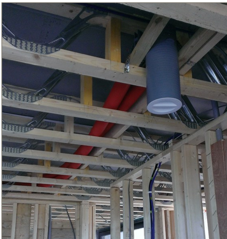
Ventilation ducts running between the posi joist with outlet in the TV room downstairs.
