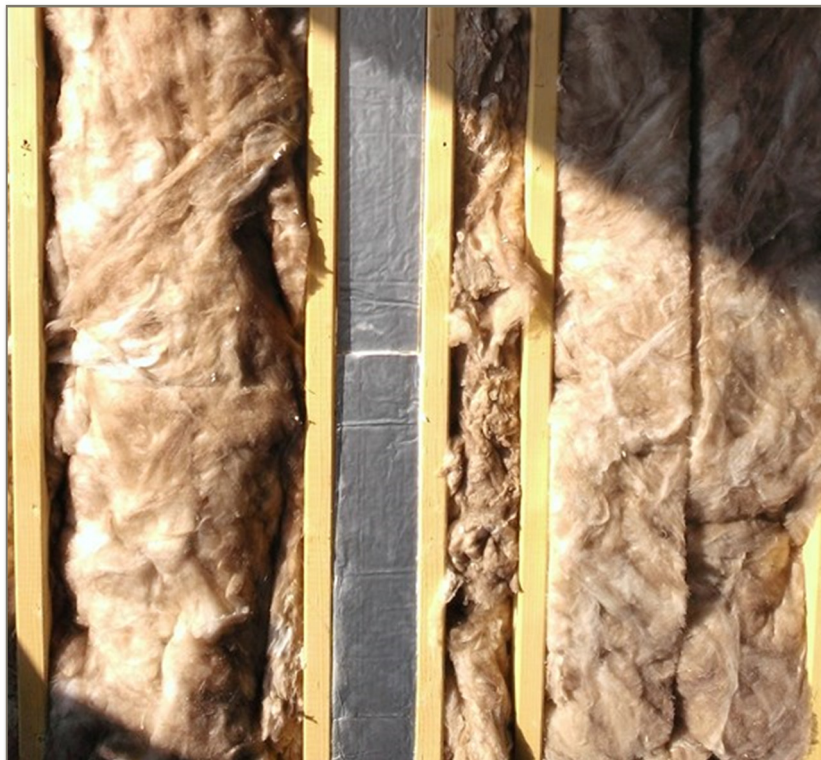
Plan detail of steel post carrying steel beam supporting blockwork moved outside thermal line to reduce thermal bridging.
