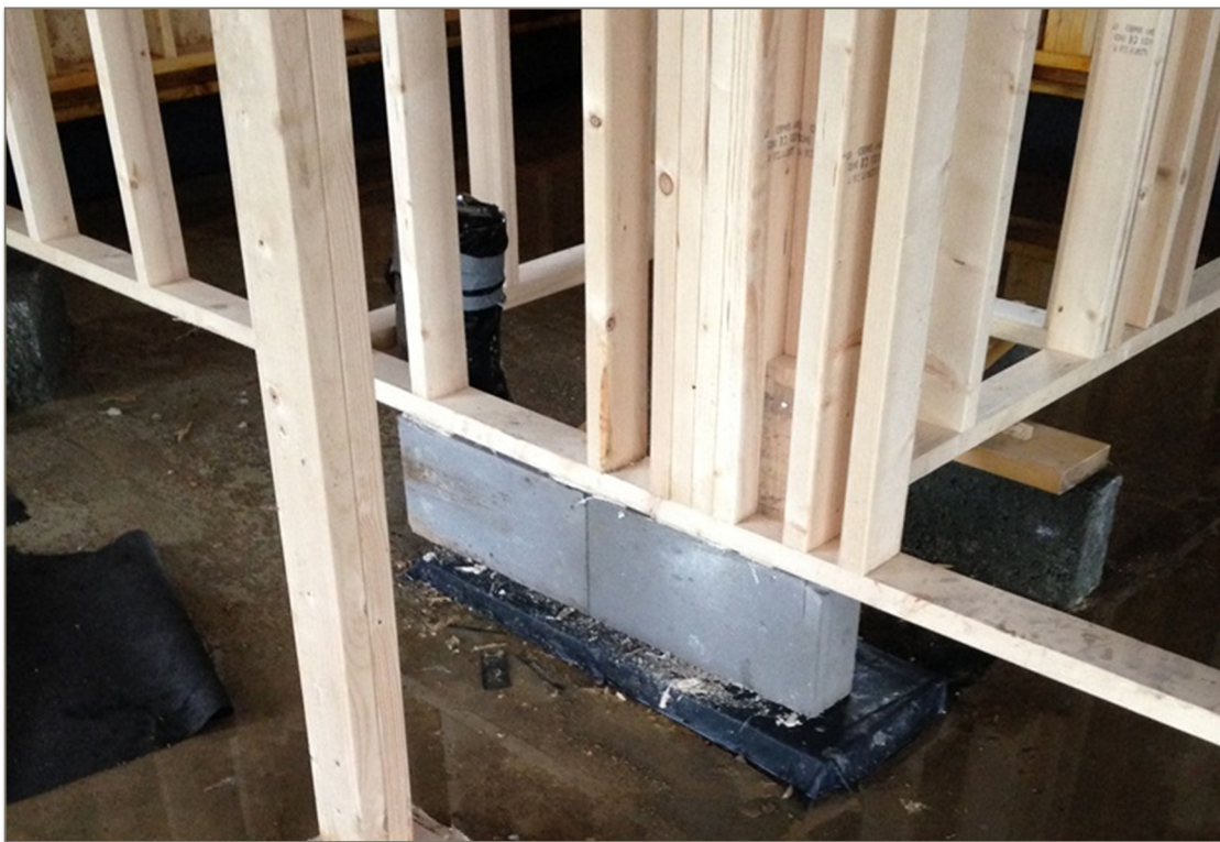
Internal load-bearing walls; QuinnLite blocks used at all penetrations through floor insulation to reduce cold bridging.
