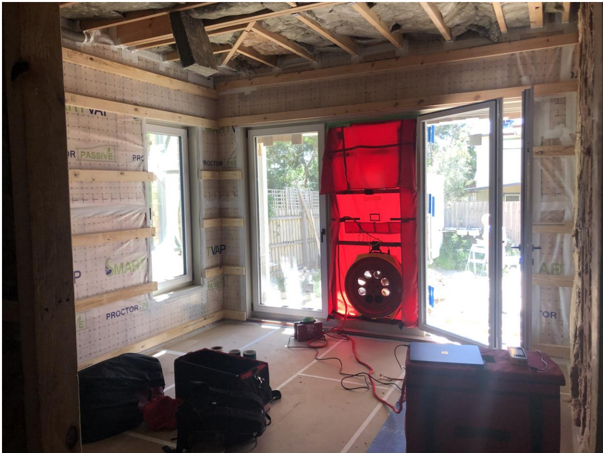
A test conducted, pre-plaster from the North-East bedroom of the Ground Floor
