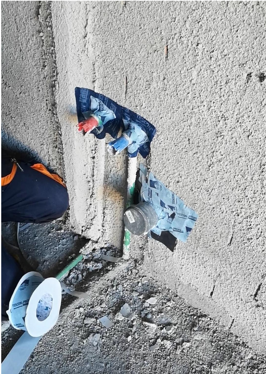
Picture 14. Sealing collars on ducts
