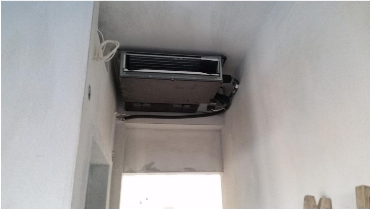
Picture 18. Split unit air condition at the 1 st floor
