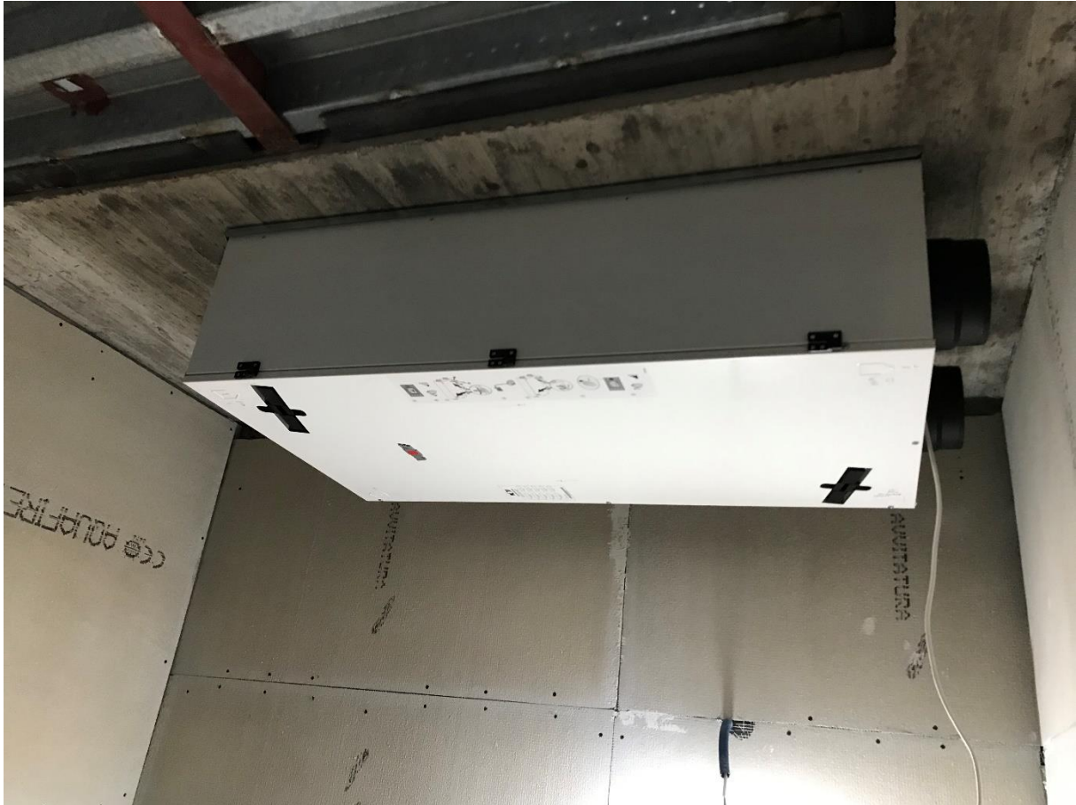
Picture 42: Ventilation unit, ground floor
