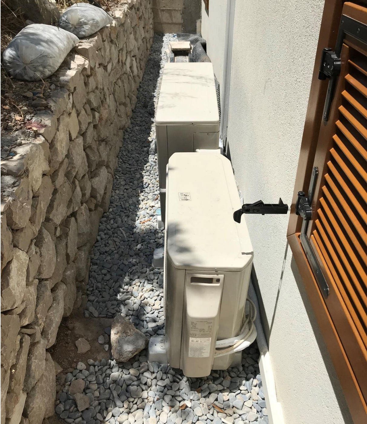
Picture 43: Air to air heat pumps outdoor units for heating and cooling.
