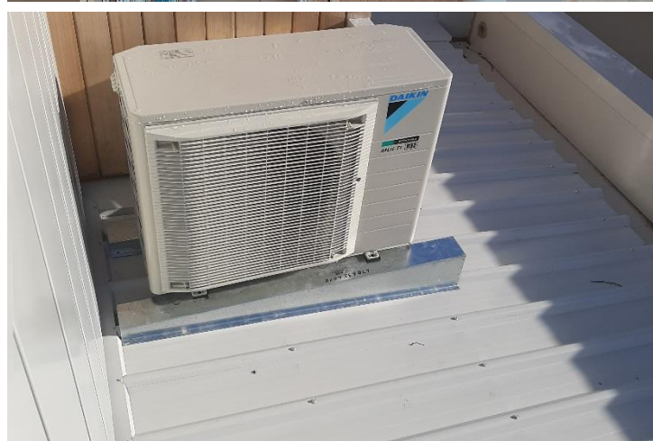
Typical indoor A/C head and upstairs air-to-air heat pump on roof
