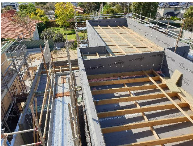
Flat roof sections under construction; CLT parapet in grey WRB and mineral wool installed below battens in distant roof
