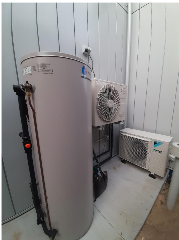
DHW storage tank and heat pump, with air-to-air heat pump across back wall (right of image).
