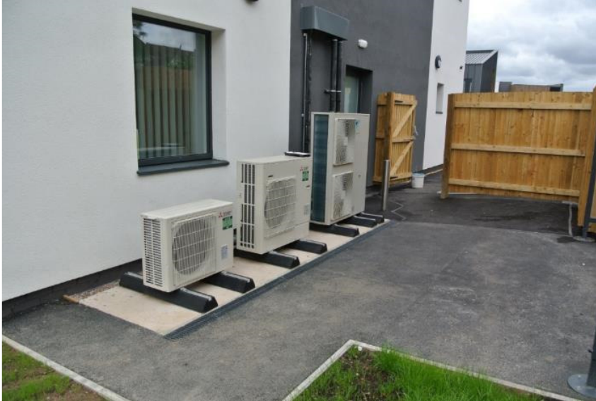
Rear elevation facing north. Note heat pump and air conditioning units and discreet rear access for staff.
