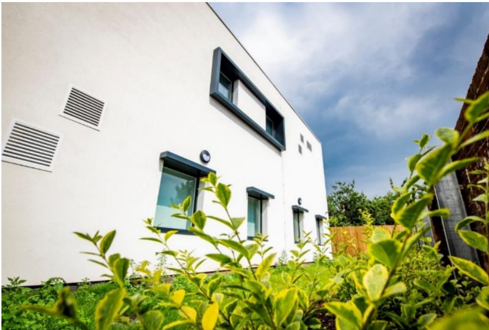
East facing elevation toward garden Ground floor consulting rooms face private garden area Note MVHR inlet and discharge terminals on clean side of the building (not to car park)
