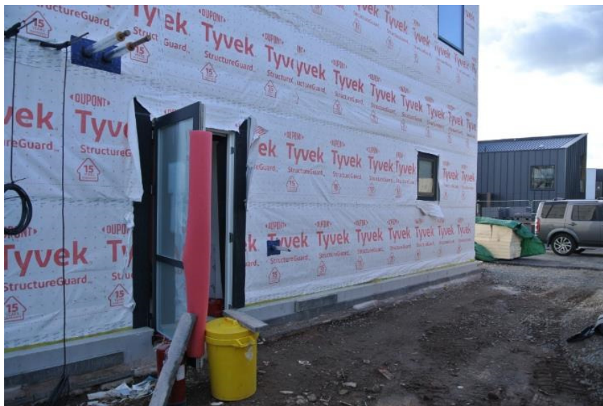
Rear elevation external wall during construction – note airtight layer and air sealing at heat pump pipework
