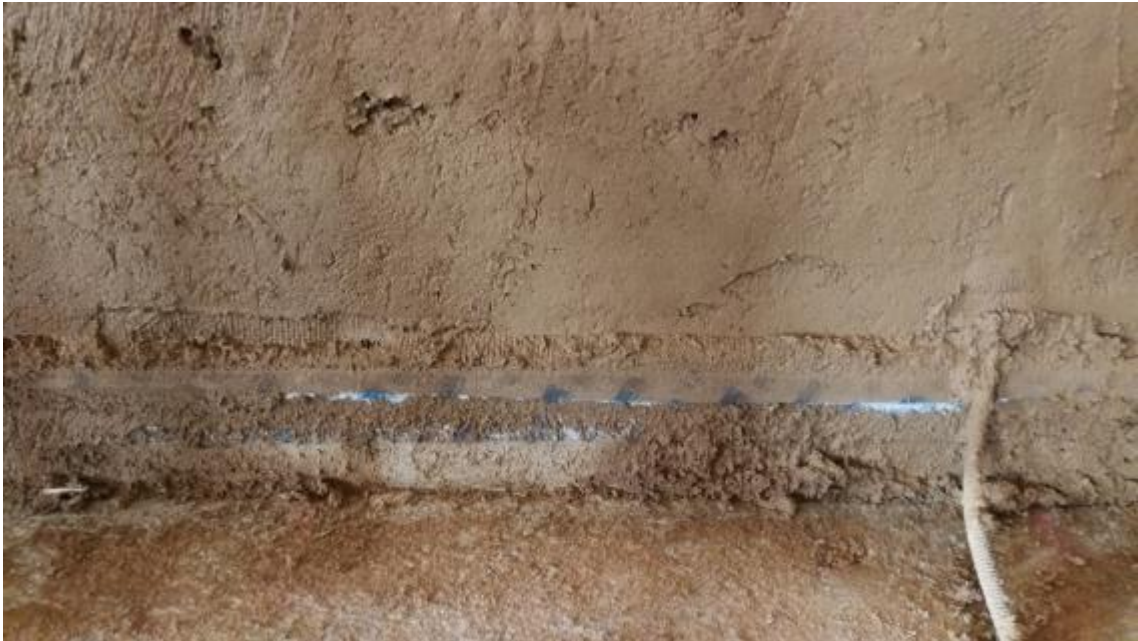
Clay plaster and connection of the airtightness sheets and tapes on the floor
