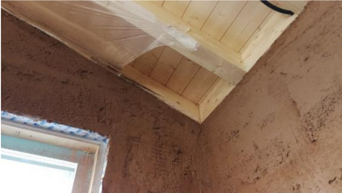
Clay plaster and connection of the airtightness sheets and tapes on the window and roof
