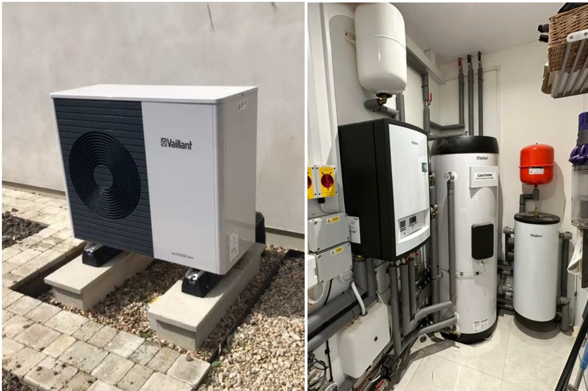
Fig. 10: Vaillant Arotherm monobloc ASHP (left) and plant room (right) containing Vaillant indoor hydraulic module, DHW store and 45 litre buffer vessel.
