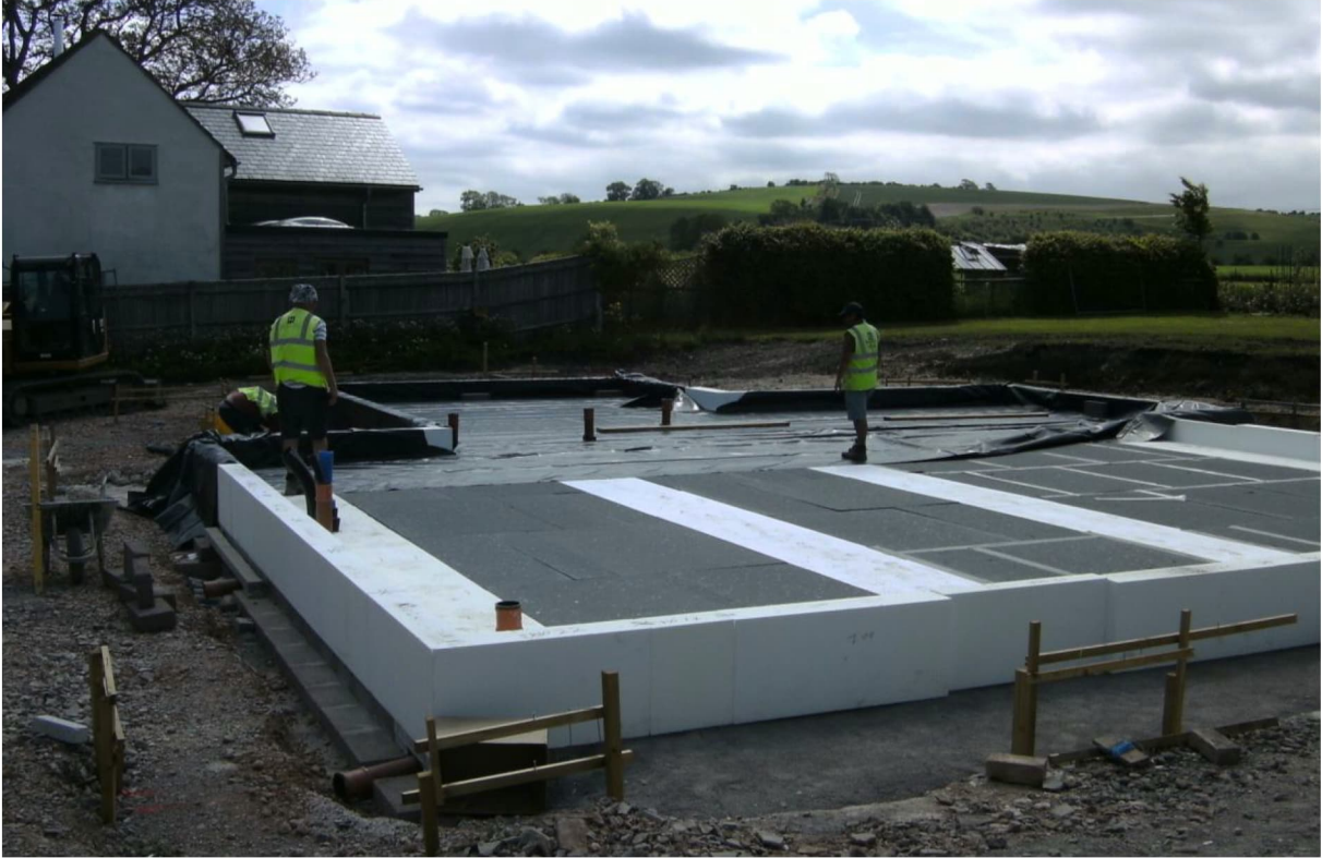
Fig. 1: First 200mm layer of EPS insulation being prepared with DPC before installation of second 200mm EPS layer.
