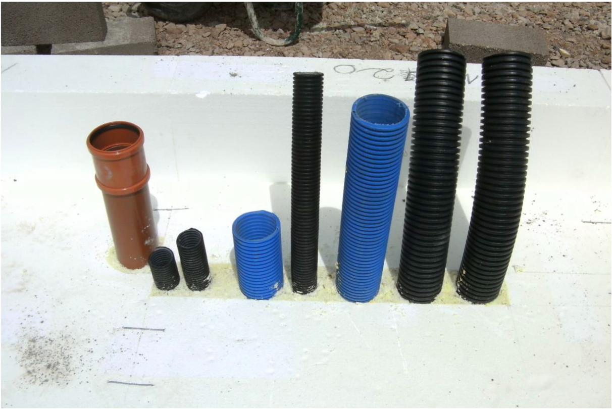
Fig. 2: Plant room service penetrations entering via pre-ducted routes in the ground floor slab.
