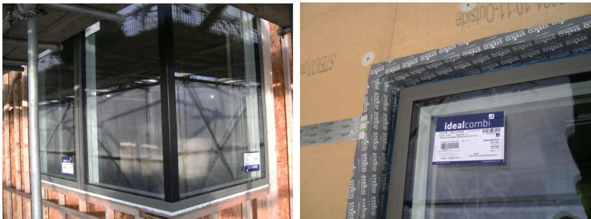
Fig. 7: Ideal Combi aluminum composite windows before (left) and after (right) installation of external woodfibre insulation.
