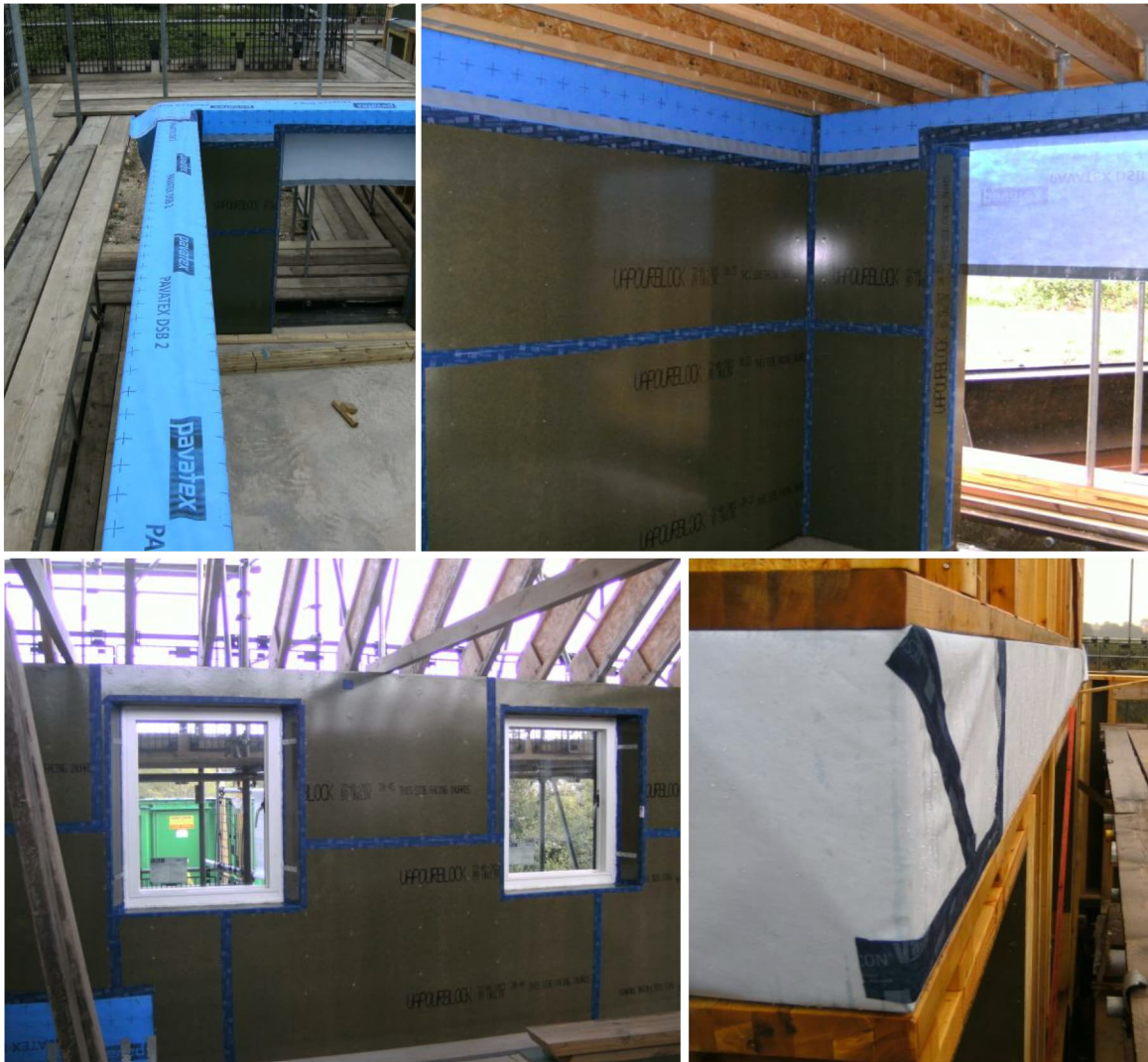
Fig. 8: Airtightness membrane taped and lapped over mid-floor joists, and window frames installed within airtight layer using flexible airtight expanding foam.
