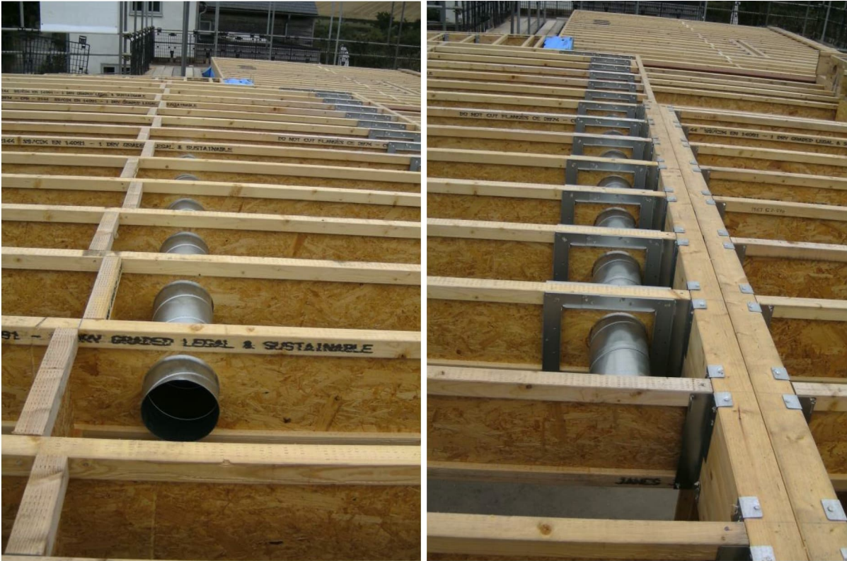
Fig. 9: Installation of rigid steel spiral wound ventilation ductwork in mid-floor joists for distribution of supply and extract air to ground and first floor rooms.
