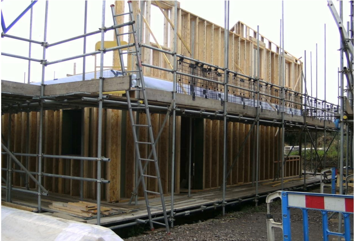
Fig. 3: Timber I-Joist frame in construction. The airtightness membrane wrapped around the mid-floor joists can be clearly seen.
