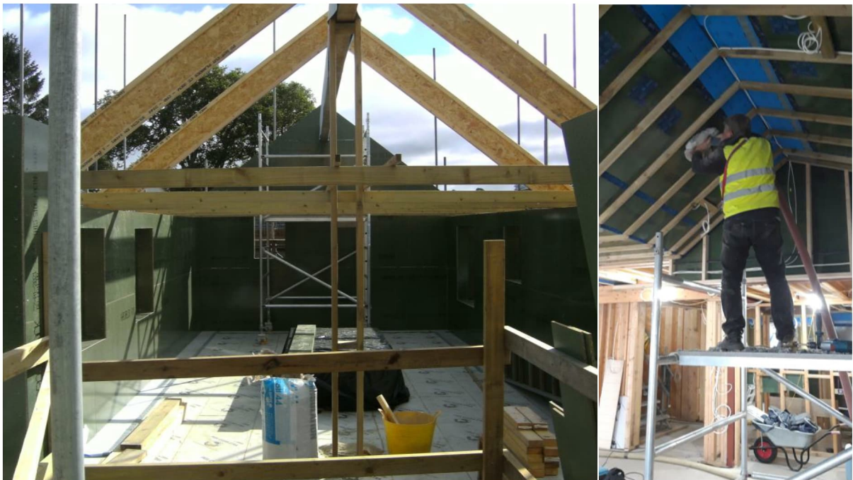
Fig. 6: Timber I-Joists spanning to glulam ridge beam (left) and installation of blown cellulose insulation (right).
