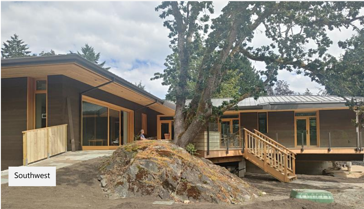
Patio deck and unfinished yard to southwest of building, including retained central Garry Oak tree.
