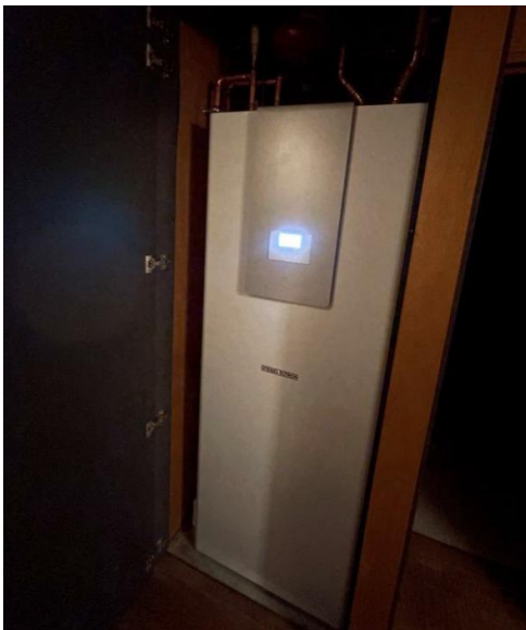
Hot water unit
