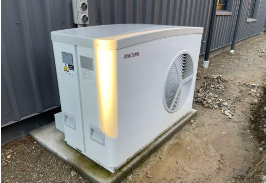
Heat pump exterior unit
