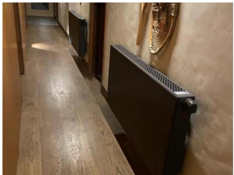
Example of radiator
