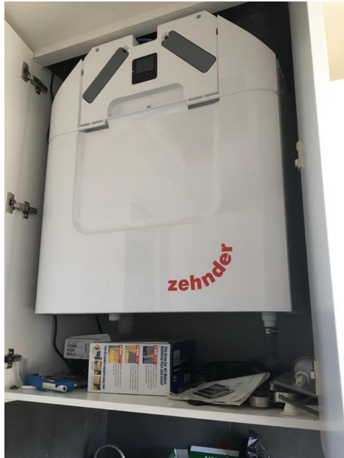
Heat Recovery Ventilation system
