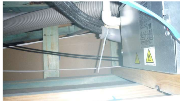
INTERIOR SPACE HEATING UNIT IN CEILING BULKHEAD
