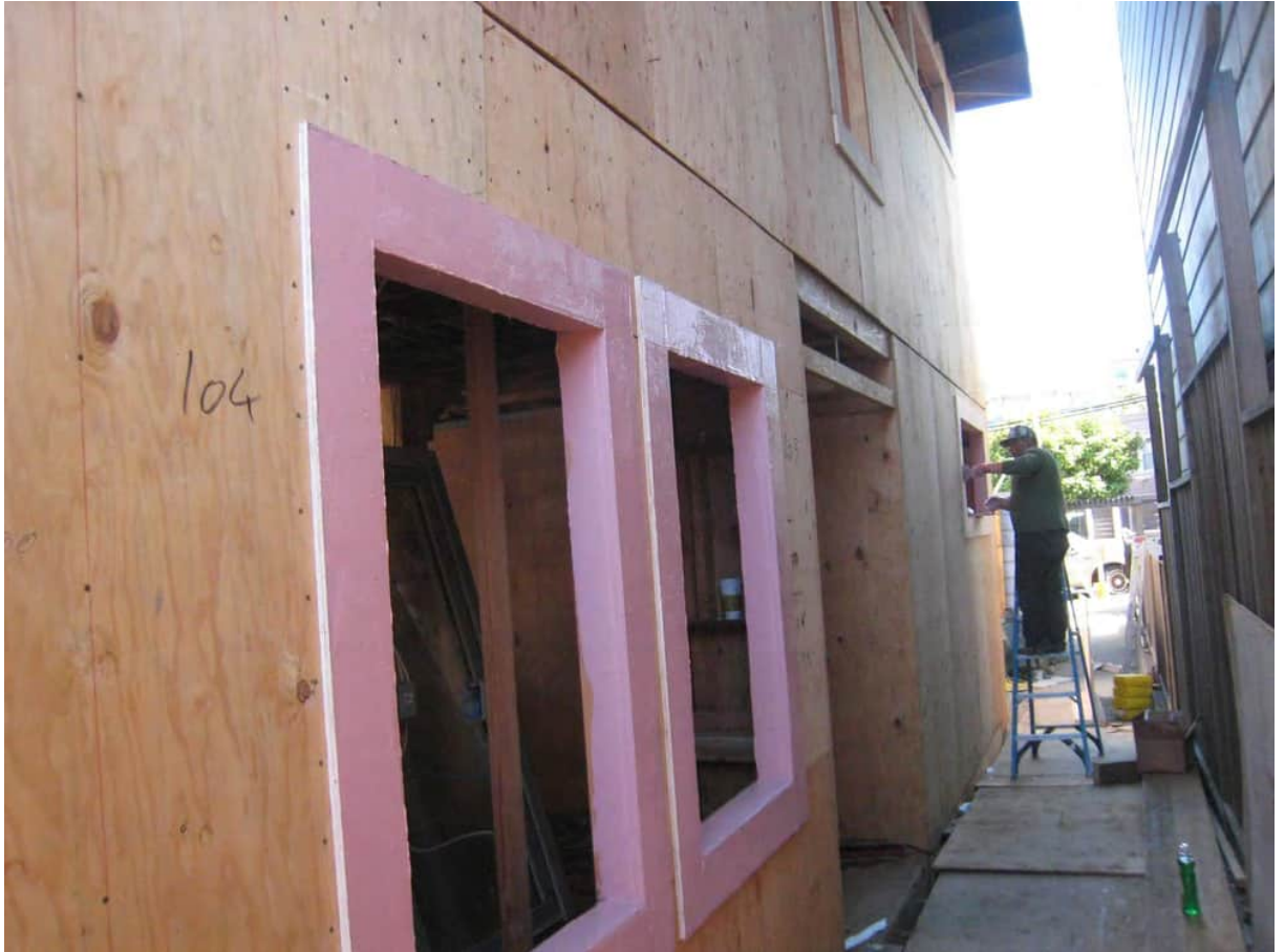
Photo of Window Rough Openings, West Wall, prepped with Liquid-Applied Air Sealant
