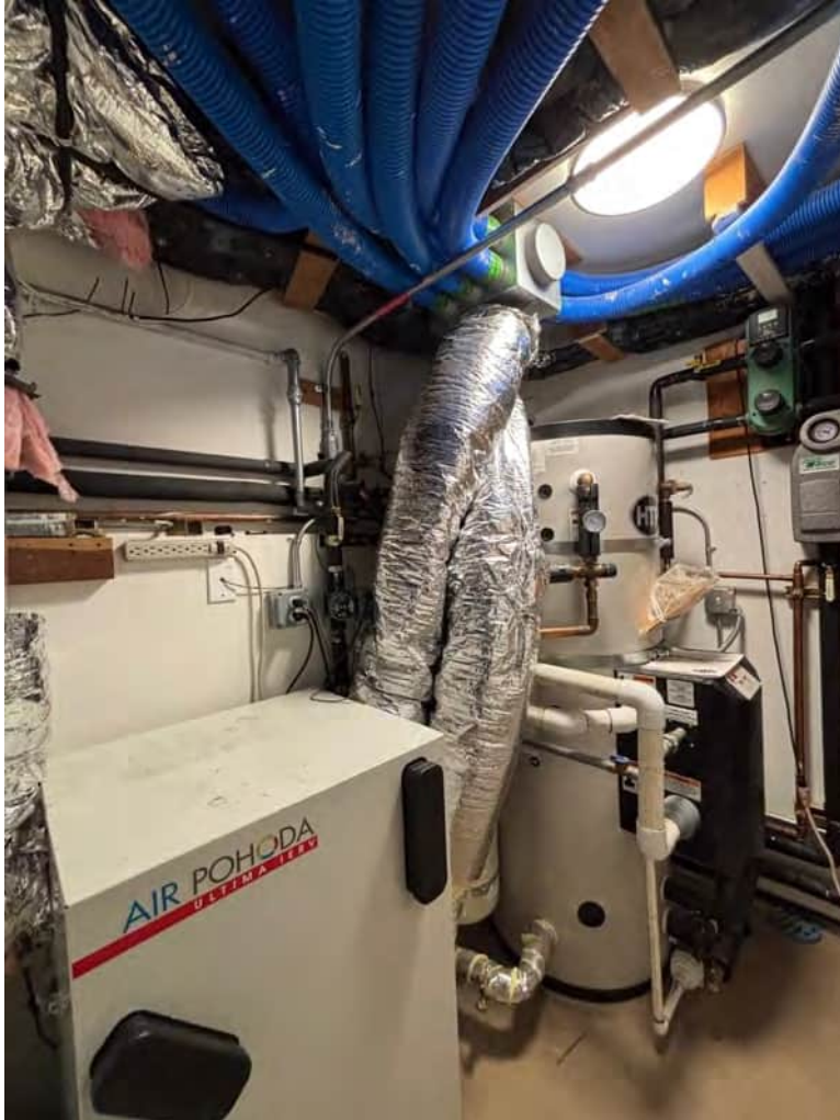
Ventilation Unit, Adjacent to DHW Cylinder & Boiler
