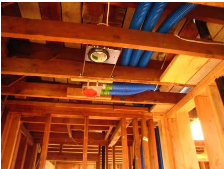
Extract Air Ducts
