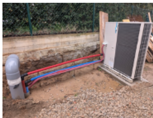
Exterior unit of the Panasonic heat pump
