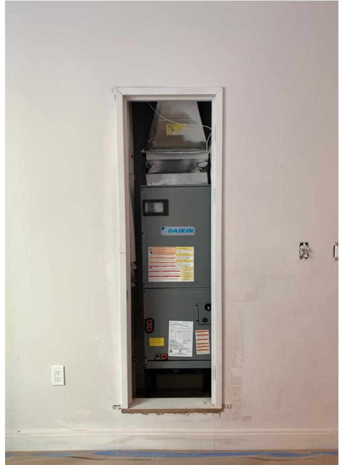
The indoor evaporator units fit nicely into closets within each apartment.
