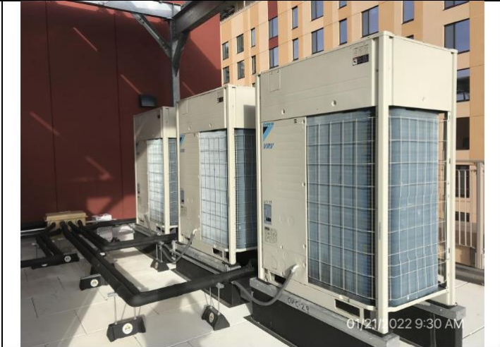
Notes: Overview outdoor units on 10 th floor east side roof
