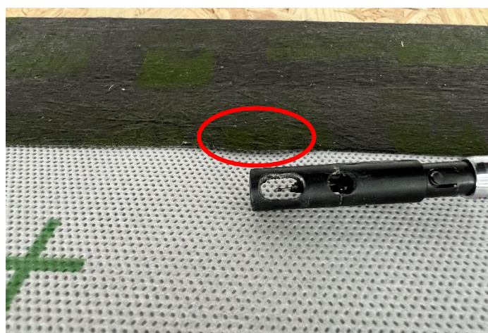
Fig. 12: Leakage measurable with an anemometer at the transition between membrane and adhesive tape before rework. Leakage detectable only at higher pressures
