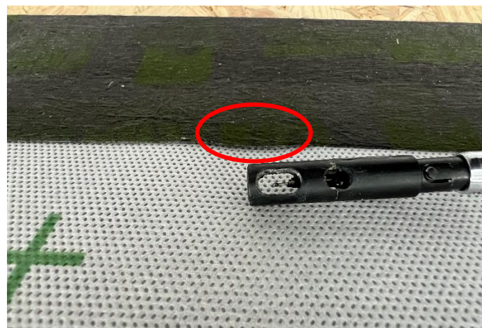
Fig. 12: Leakage measurable with an anemometer at the transition between membrane and adhesive tape before rework. Leakage detectable only at higher pressures
