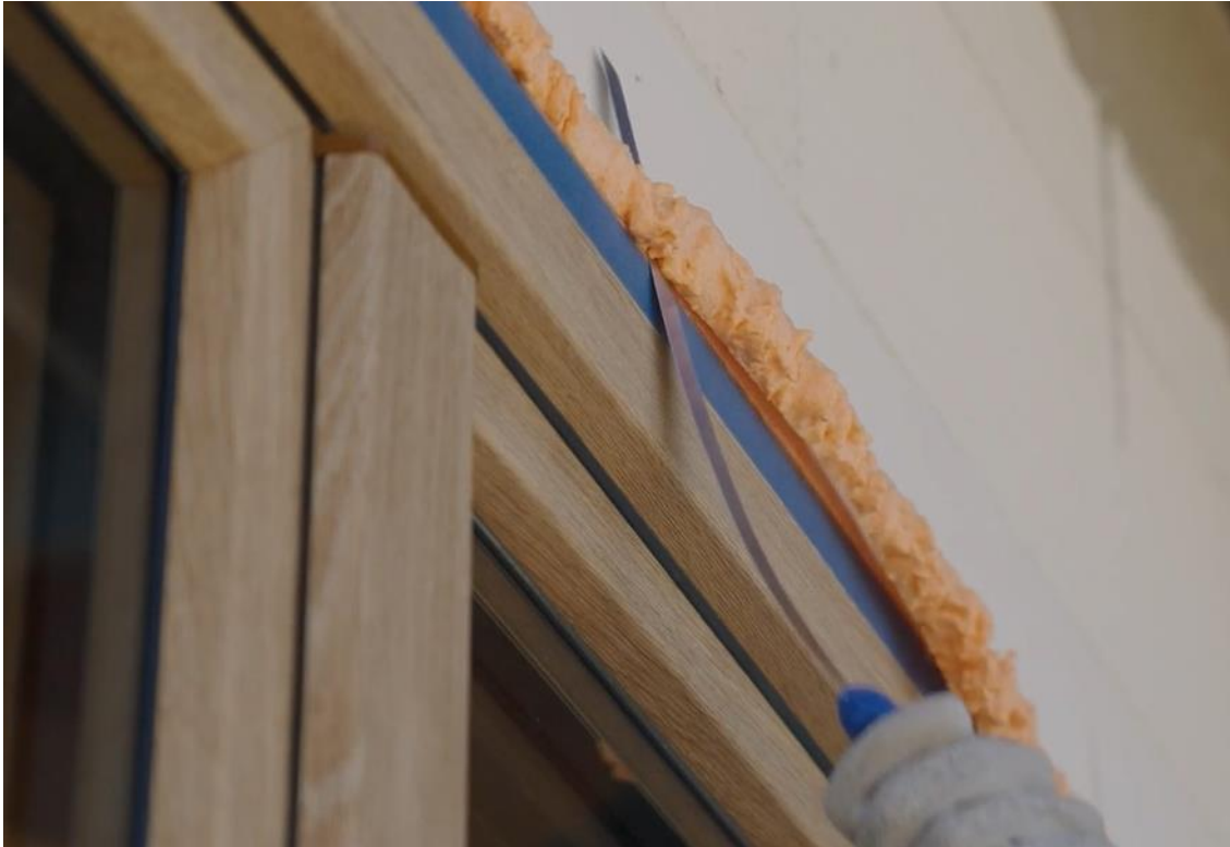
Picture no 12. During cutting the cured pu foam, is possible bend the blade without deformation
