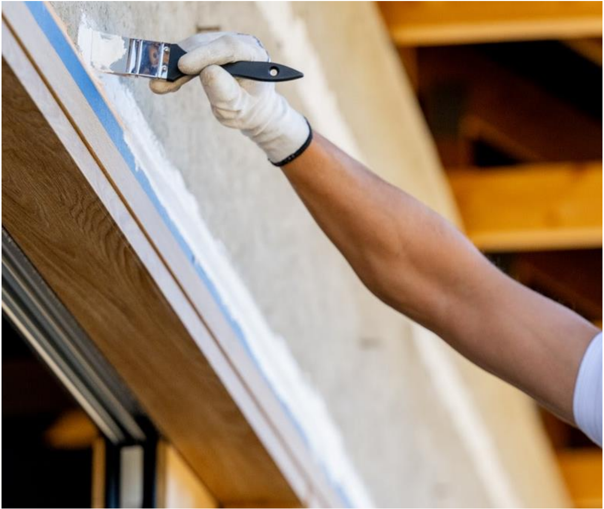
Picture no 16. Application external liquid foils by TYTAN silicone applicator from outside
