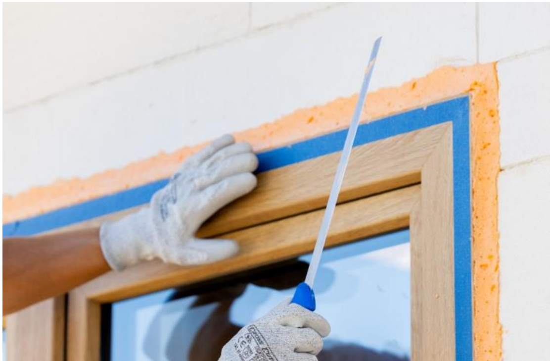
Picture no 14. After cutting the cured pu foam is visible smooth line, window between frame – outside line of the wall or dedicated warm beams (for example MARBET beams) in case passive houses
