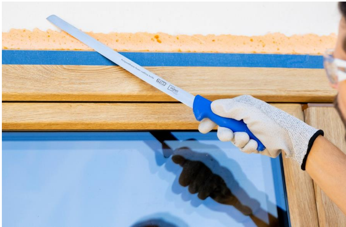
Picture no 13. After cutting the cured pu foam is visible smooth line, window between frame – outside line of the wall or dedicated warm beams (for example MARBET beams) in case passive houses
