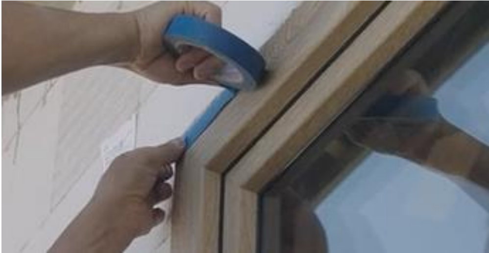
Picture no 3. Protect the surface of the joinery by masking tape from both sides
