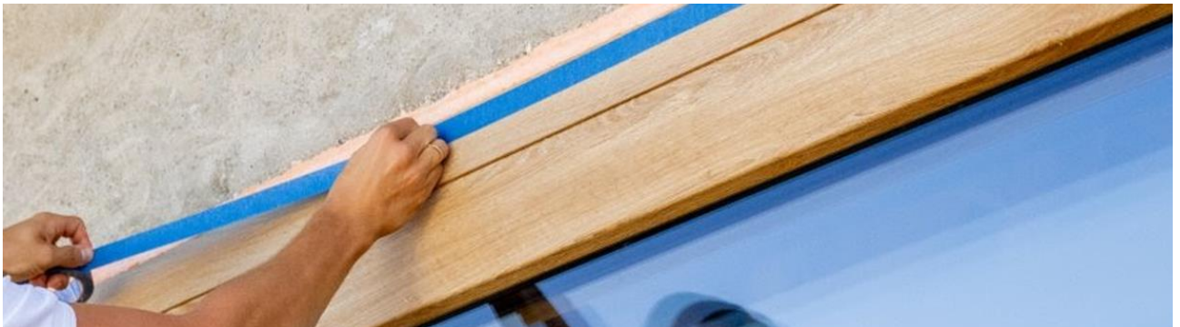
Picture no 2. Protect the surface of the joinery by masking tape from both sides
