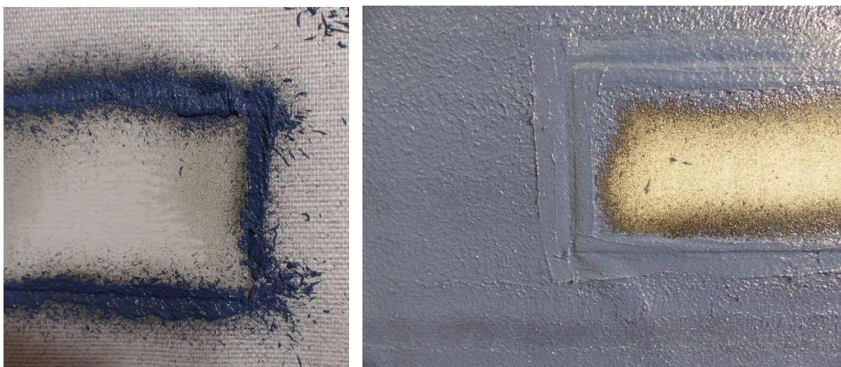
Fig 5: Filling the gap around the concrete slab (left) and situation after applying the surface seal around the concrete surface (right).
