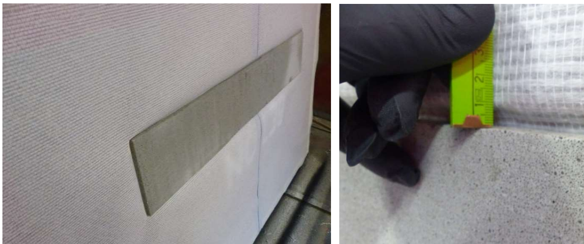
Fig 4: Inserted concrete slab (left) and size of the remaining gap (right).
