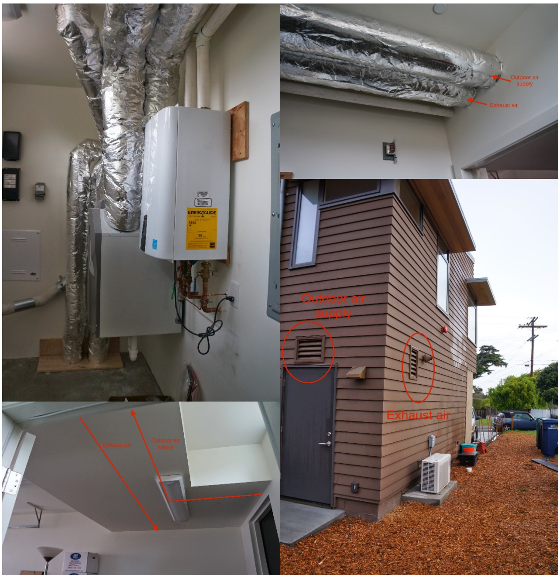
Figure 17 Marked images of the heat recovery ventilation system, Zehnder ComfoAir 350 (top left), duct work from HRV into drop ceiling in garage (top right), location of ducts in drop ceiling (lower left) and outside termination/supply points (lower right).
