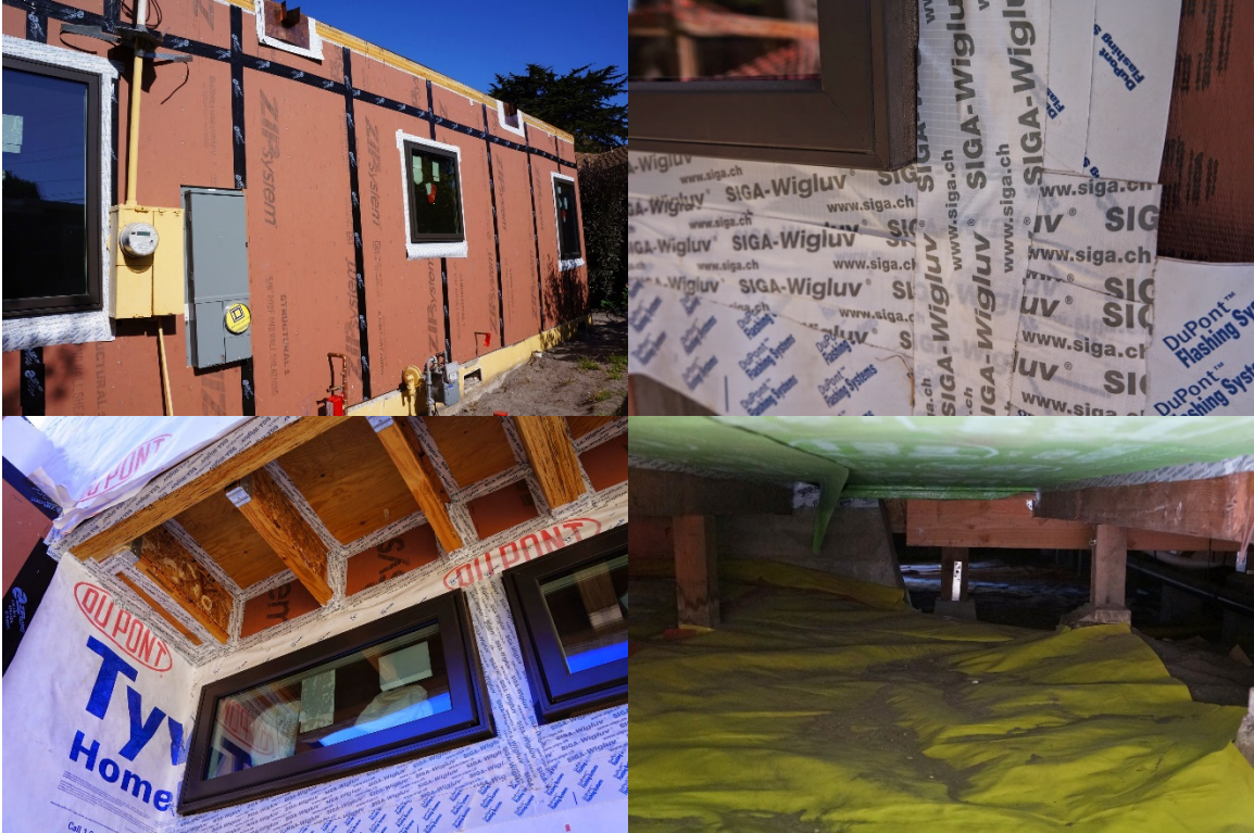
Figure 13 Air sealing details for a typical exterior wall (top left), a window (top right), an exposed floor (lower left) and the existing floor with crawlspace (lower right).
