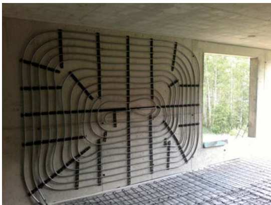
Photo 16.- 39/33° C supply/return temperature
