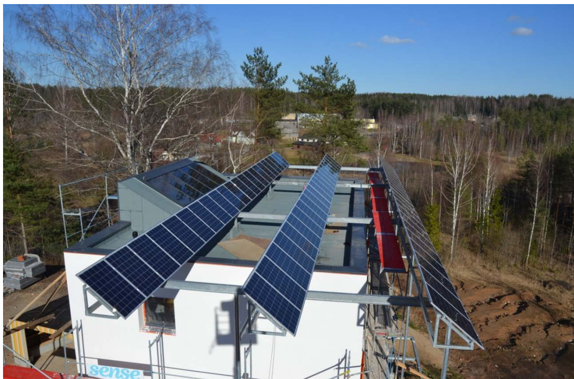
Photo 18.- PV on the Roof and Solar thermal collectors on the left.
