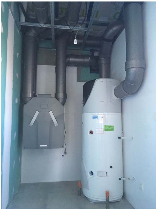
heat recovery and the heat pump
