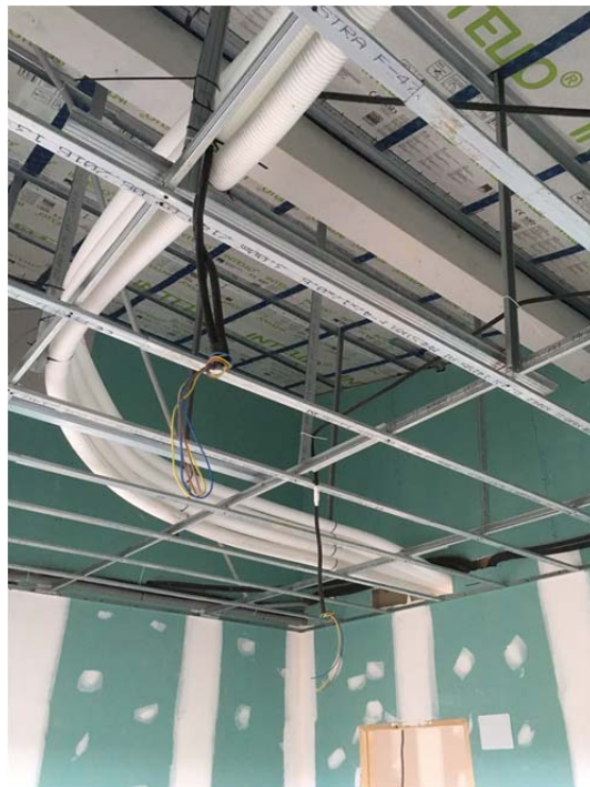
ventilation ducts over the ceiling
