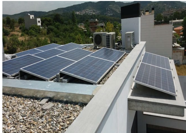
Photovoltaic plates on the roof
