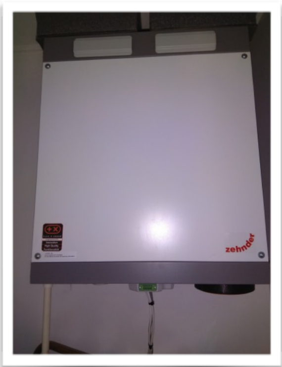
Zehnder ComfoAir 180 HRV unit installed on the secondary dwelling
