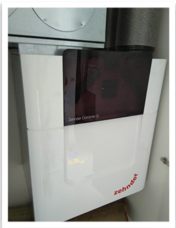
Zehnder ComfoAir Q600 HRV unit installed on the main dwelling
