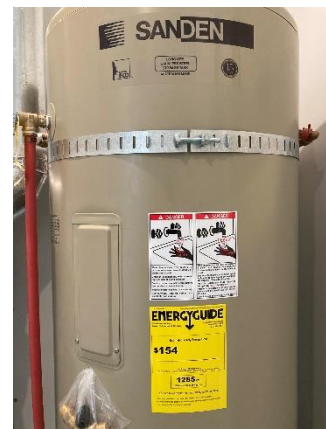
Interior Insulated Tank
