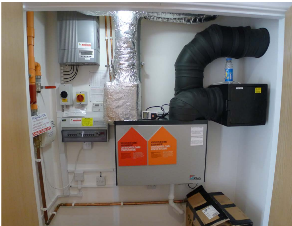
Figure 18. Showing the Paul Focus MVHR unit and preheater and pre-filter box (black polystyrene) and insulated post heater and risers (wrapped in foil-faced mineral fibre)
