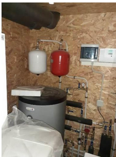
Domestic hot water tank
